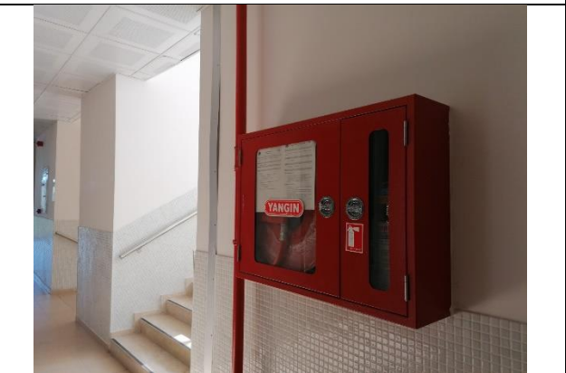
Equipment in all buildings
