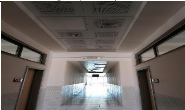
Fire sensors, automated security system
