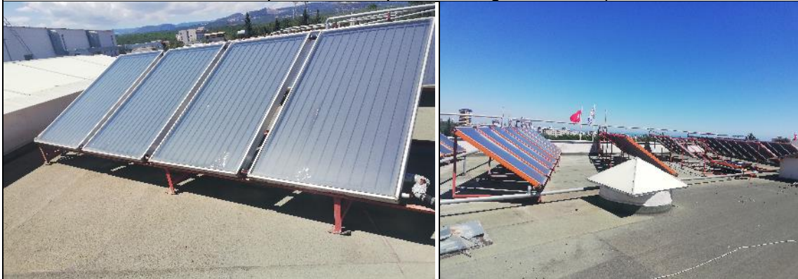
Examples of Energy Efficient Appliances Usage: Solar absorption system (Mersin University, Turkey)
