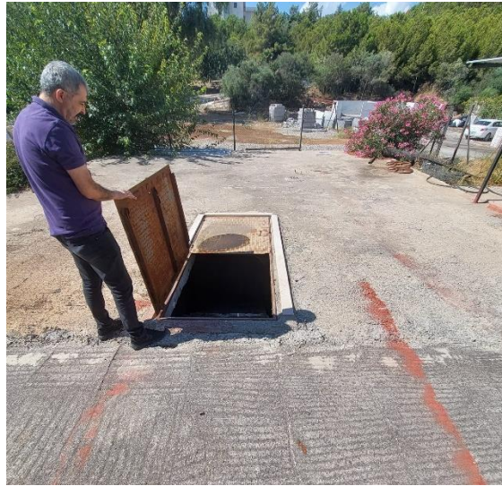
Rainwater Harvesting System - Cistern (water reservoir)
