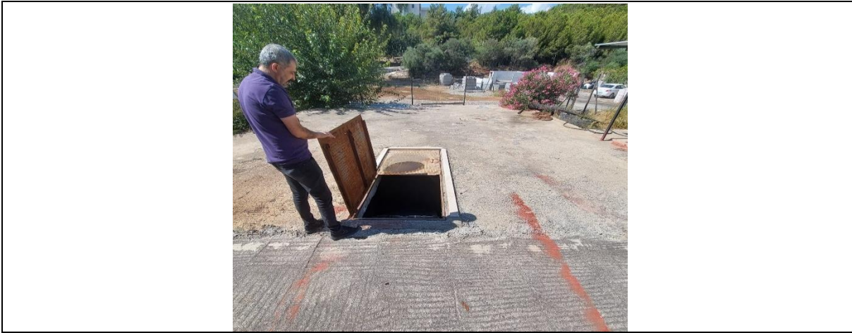
water booster for irrigation - Cistern (In Ground Water Tank)
