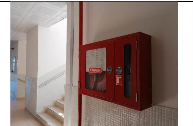
Equipment in all buildings
