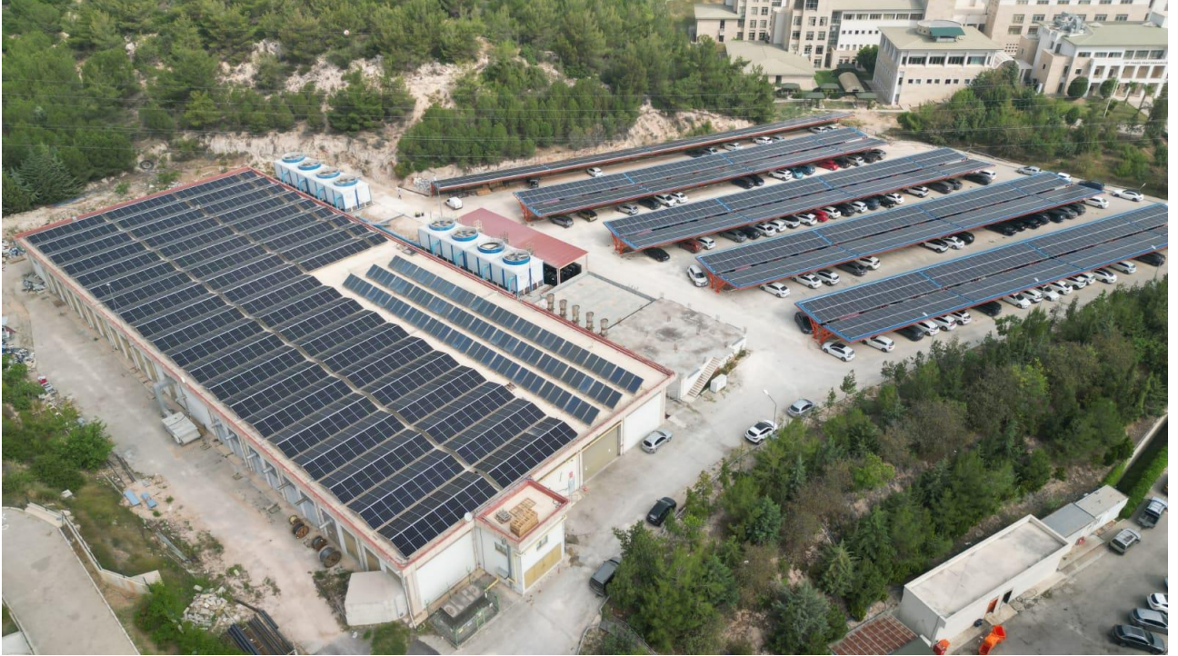
Renewable energy simulation software and installation of renewable energy
