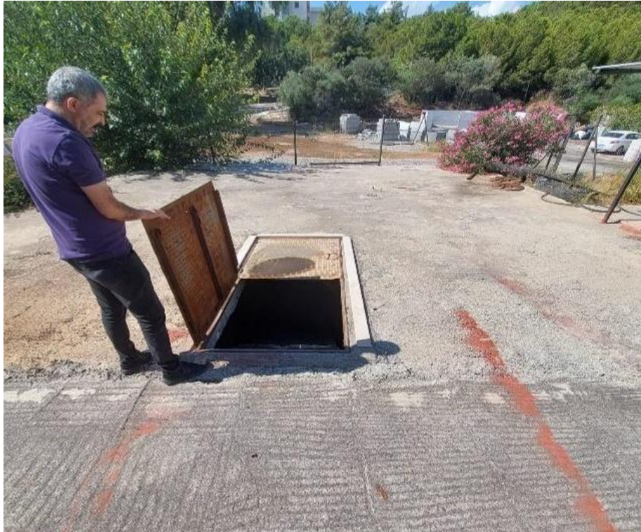
water booster for irrigation - Cistern (In Ground Water Tank)
