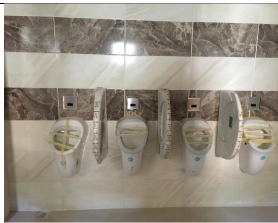
LEDs, energy efficient automated and motion sensitive
