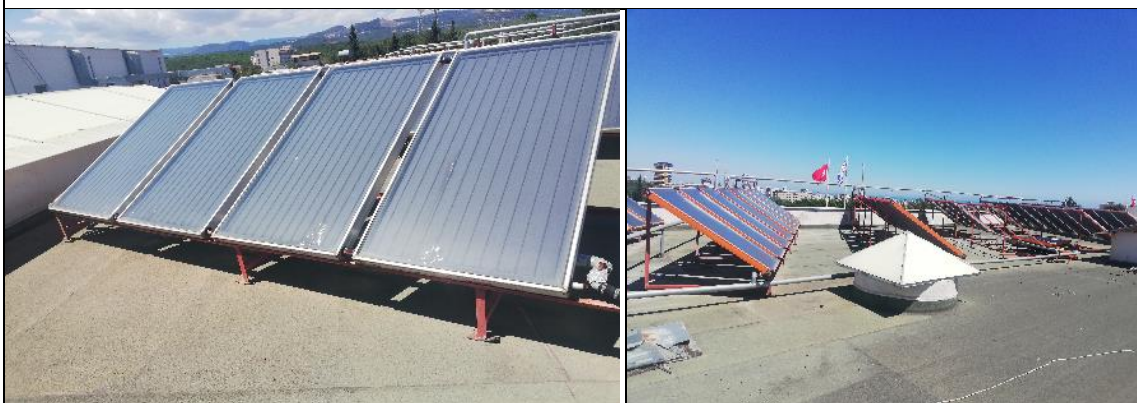
Examples of Energy Efficient Appliances Usage: Solar absorption system (Mersin University, Turkey)
