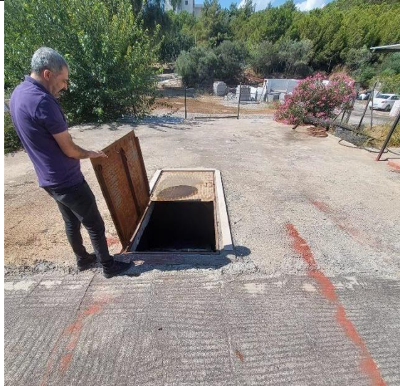
Rainwater Harvesting System - Cistern (water reservoir)
